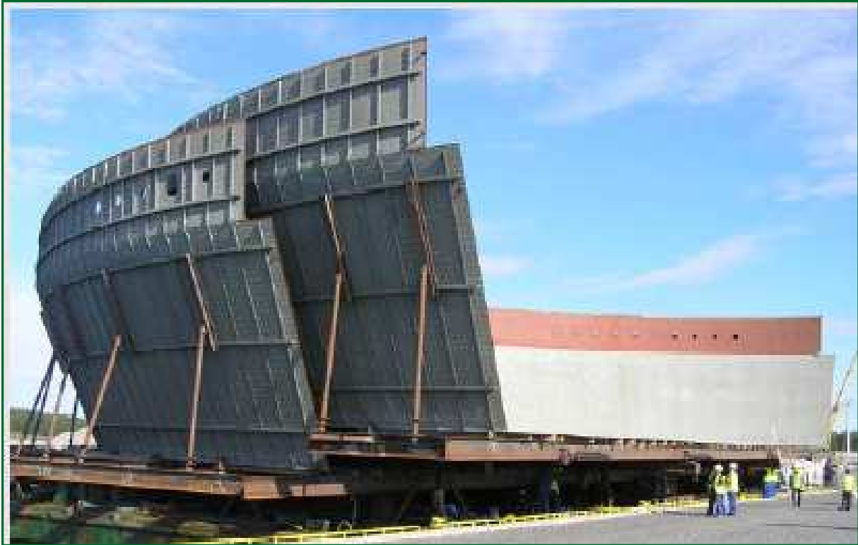
Figure 2 The behavior of this containment steel liner at Olkiluoto 3 was also verified with ATENA software.
